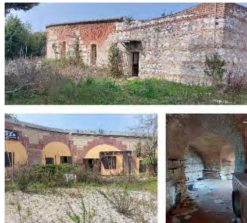
Fig.4- Forte Scrima. Main building, which housed a restaurant until 2020, with the inner courtyard and rooms severely damaged
